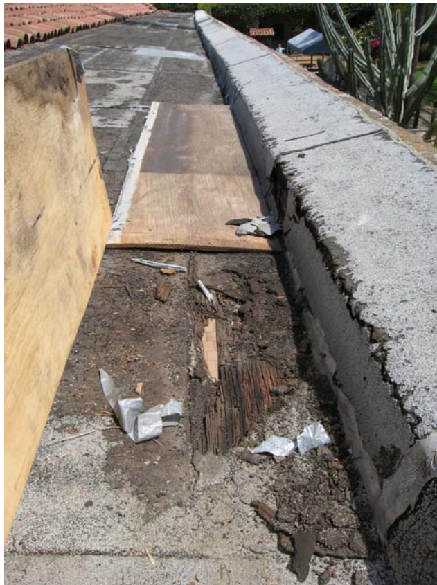
Before Water Intrusion Damage
