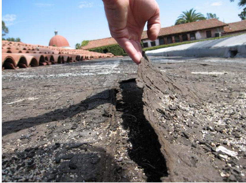
Before Deteriorated Roof Membrane
