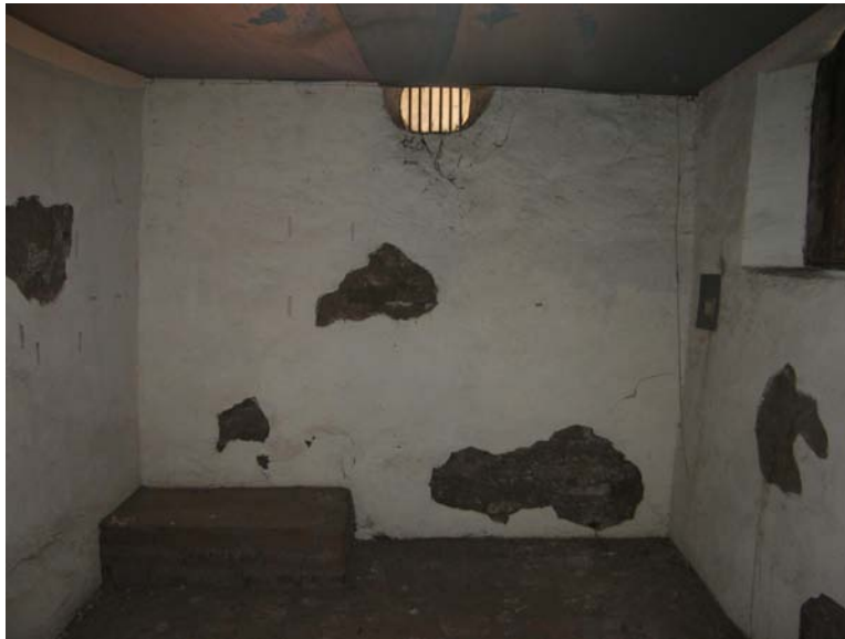
Before Southern Dormitory wall before treatment
