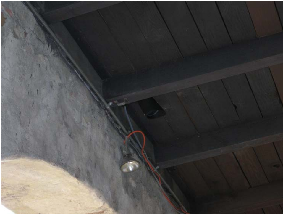
Mission Arcade Lighting Project New replacement low profile light fixture next to existing fixture
